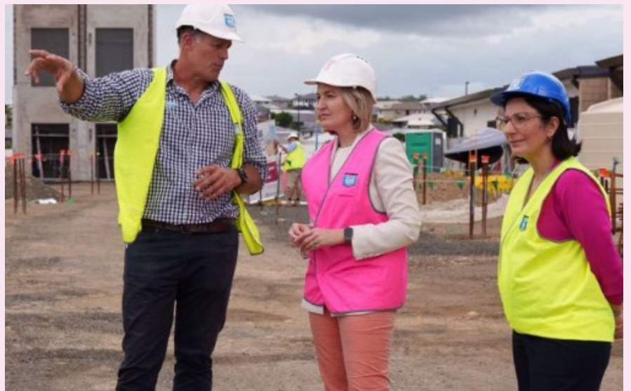
Hutchies' team leader, Jamie Washington, updates Queensland Minister for Health, Shannon Fentiman (centre), and local MP, Charis Mullen, on construction progress at the Ripley Sub-Acute Hospital site.
