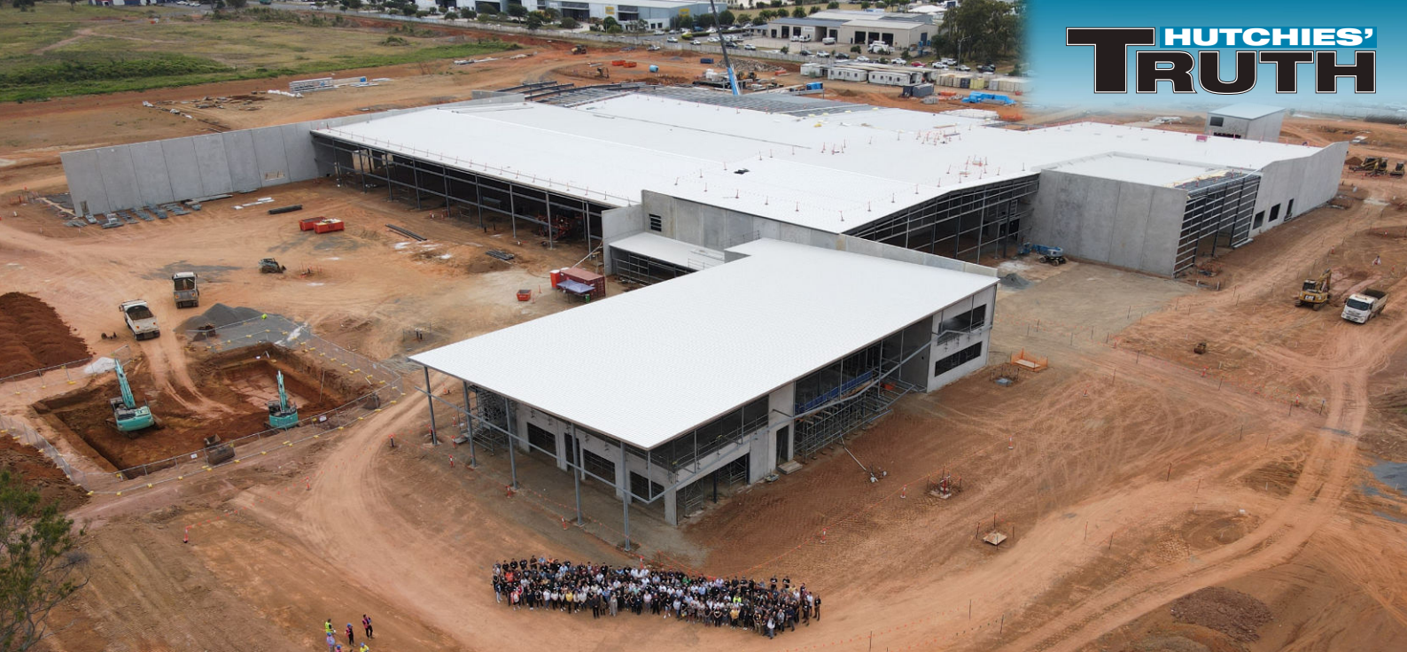
Bundaberg Brewed Drinks' 200 staff members visit the company's new brewery being built by Hutchies in Bundaberg.
