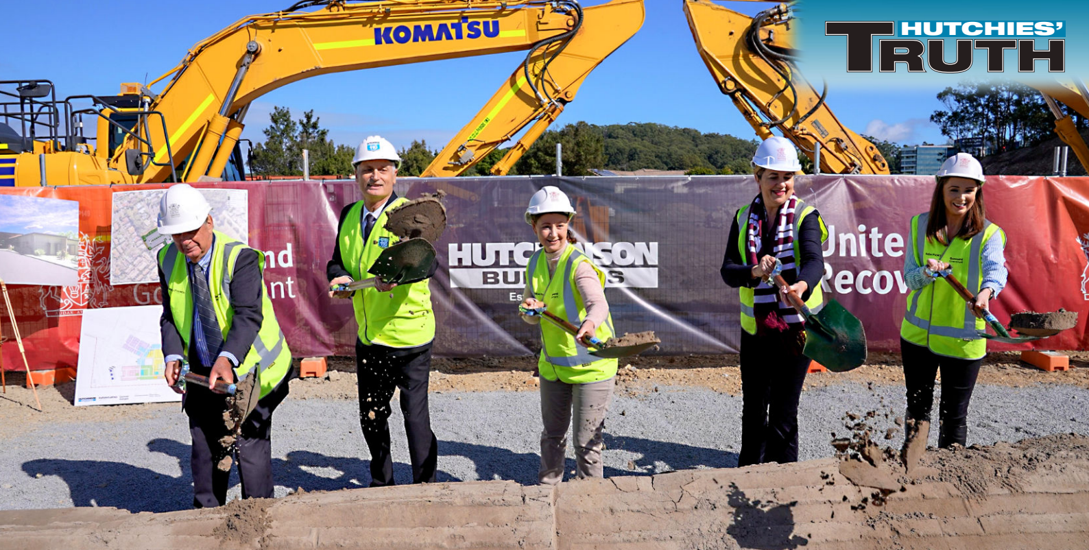
Sod-turning for the new Gold Coast satellite hospital at Tugun – one of the seven new hospitals under construction by Hutchies for the Queensland Government’s Satellite Hospitals Program. From left, chief executive Gold Coast Hospital and Health Service, Ron Calvert; Scott Hutchinson; Minister for Health, Yvette D’Ath; Premier Anastacia Palaszczuk; and Gold Coast-based Government Minister, Meaghan Scanlon.
