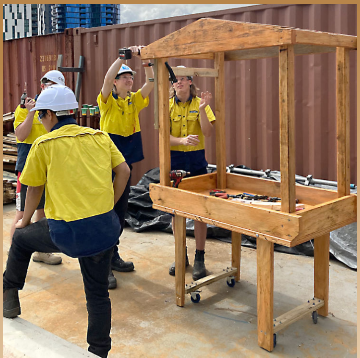
Hutchies' R4C students constructing a market cart for the West Village Market project.
