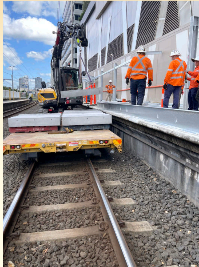
Hutchies' project team at South Bank use high rail equipment to install precast concrete coping panels to raise the platform.
