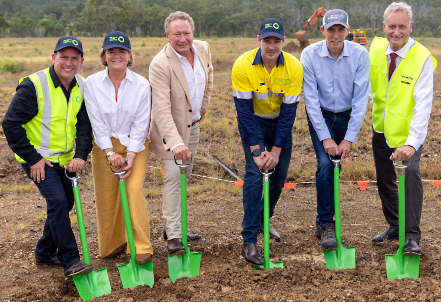
The official party signals start of work on the Gladstone electrolyser manufacturing facility, using green shovels to symbolise clean energy. They are, from left, Matt Burnett, Nicola and Twiggy Forrest, Cameron Smith, Ole Hoefelmann and Scott Hutchinson.
