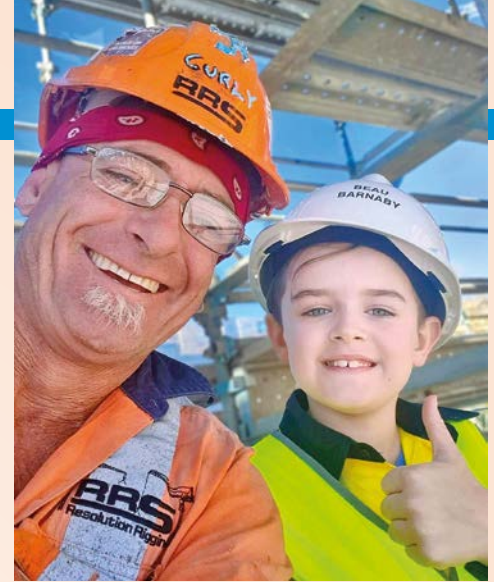
Young Beau Barnaby, son of team leader, Jayson Barnaby, recently donned his own hard hat and hi-vis and spent some time on site at PARQ on Flinders in Wollongong. Crane crew member, Jose 'Curly' Noronha from Resolution Rigging, showed Beau the ropes.
