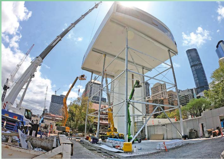
Hutchies has built the unique space age-style elevated display suite and viewing platform for the Queen's Wharf Brisbane project.
