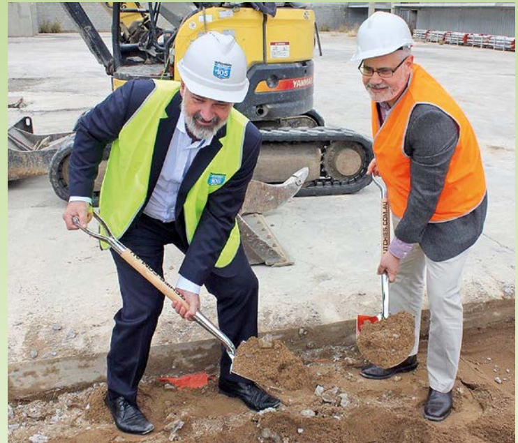
Hutchies' national construction manager, Chris Stevenson (COTY 2016), left, and Ipswich interim administrator, Greg Chemello, get to work on the new Ipswich CBD.
