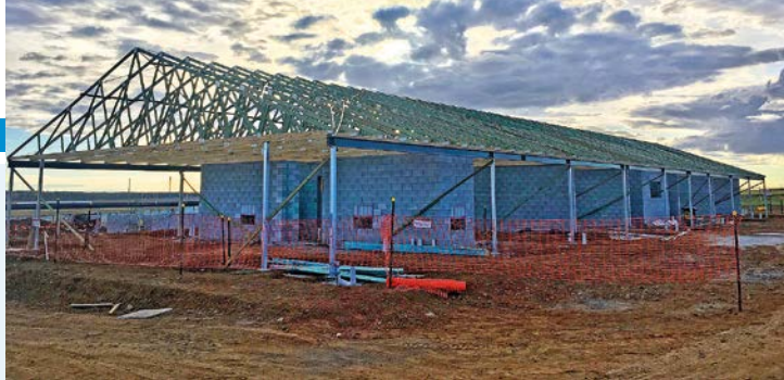
Hutchies is working on a new animal welfare care centre for the RSPCA at Wellcamp near Toowoomba.
