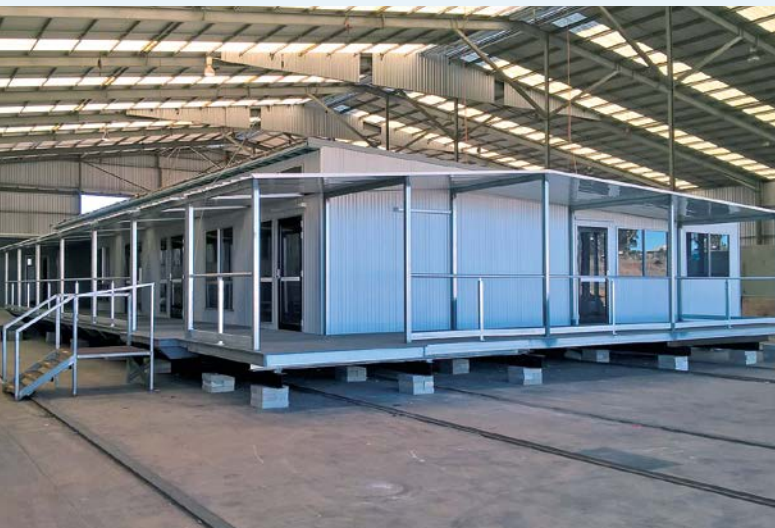
This modular build will become a new office and amenities for Aurizon in Blackwater.
