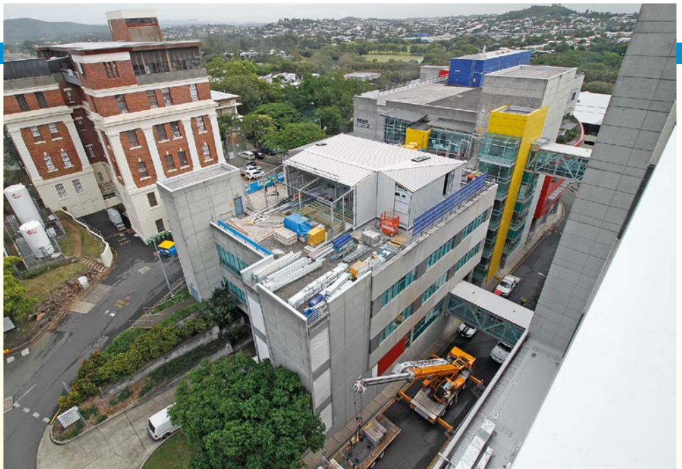
The new Sony You Can Centre atop the Joyce Tweddell building at the Royal Brisbane and Women's Hospital is nearing completion.
