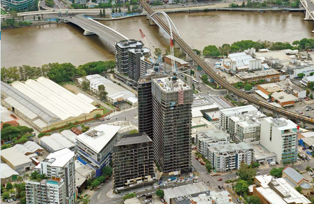
Triple-towered Brisbane 1 is a new landmark on the south side of the river city.
