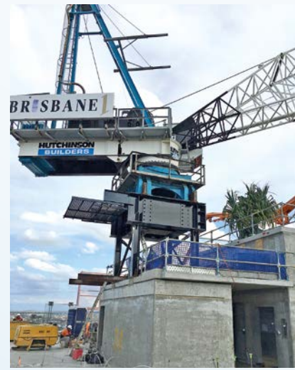
Reviving an old tradition, a tree topping ceremony was held to mark the construction milestone.
